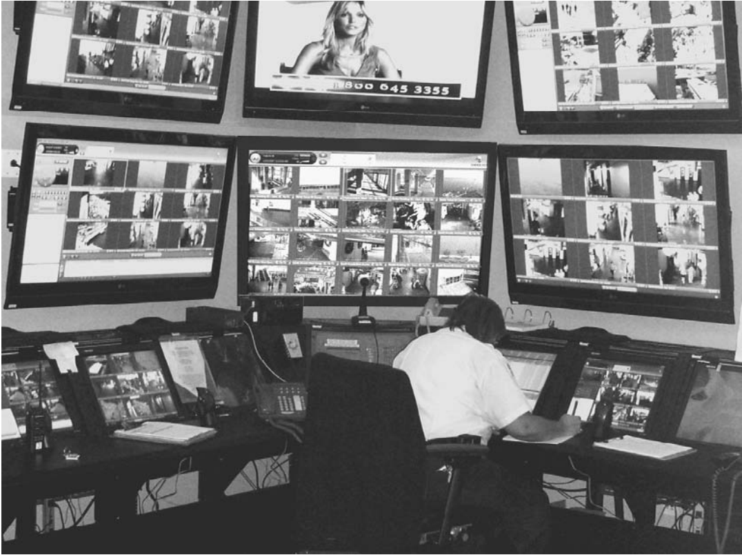
FIGURE 8-2 Navy Pier Command Center uses two dual monitor Nvidia video cards to link four 46" LCD monitors per workstation (photo courtesy of Tim Herlihy and Navy Pier).
