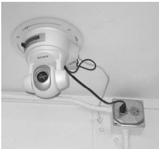
FIGURE 1-4 Avoid exposing power and data cables, providing an easy method of disabling the security camera.
