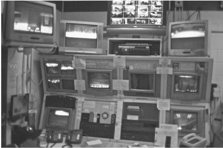
FIGURE 7-2 Before the DVS convergence there were many separate video surveillance and alarm systems running on multiple interfaces ( photo courtesy of IBM and Navy Pier ).
