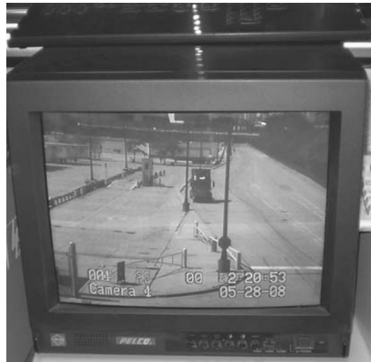
FIGURE 7-4 Typical CCTV interface, scrolling through cameras, one at a time.
