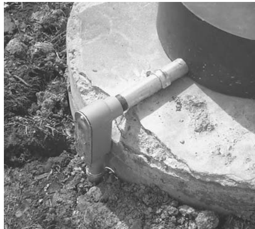
FIGURE 1-7 Exposed conduit is an easy target.
