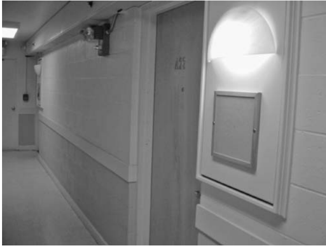
FIGURE 22.11 Interior light fixtures often use incandescent bulbs and are easy to change out, but can be subject to vandalism and produce heat gain.
