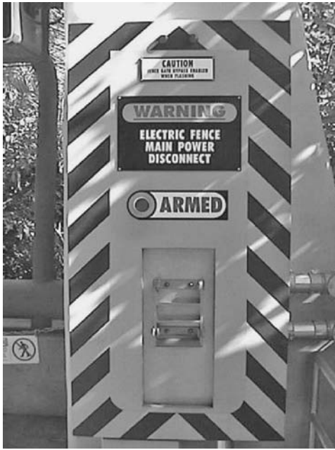
FIGURE 10.13 Signage for fences gives trespassers warning.
