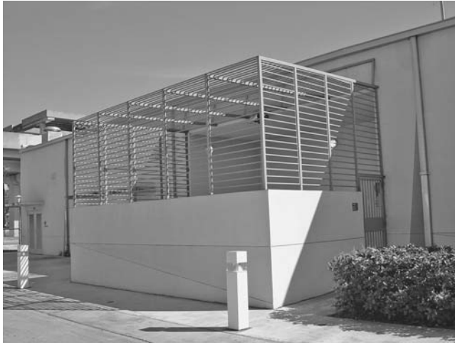
FIGURE 18.8 An exterior courtyard is covered with protective screening, but the screening acts as a ladder to the roof.
