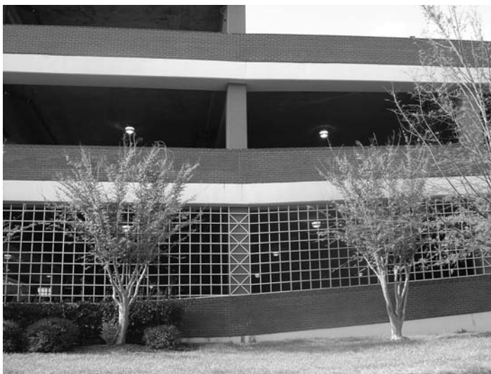
FIGURE 24.1 Ground-level protection; good intention but the screen webbing is too big and can facilitate easy climbing to the next story.
