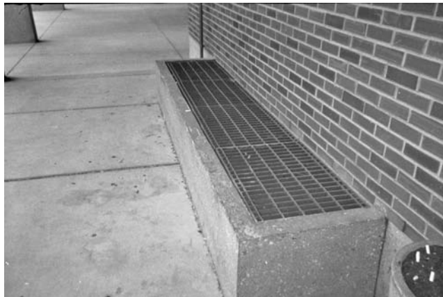
FIGURE 10.17 Air intake accessible from public walkway is extremely vulnerable.
