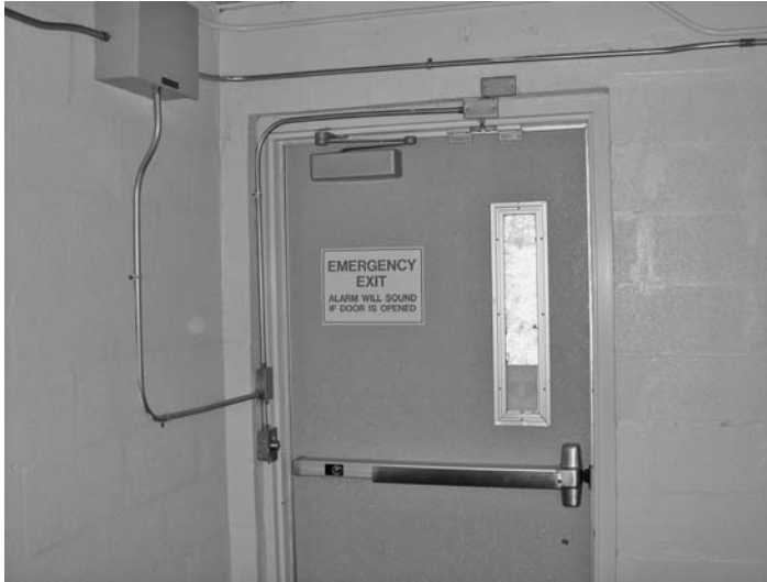
FIGURE 18.39 Retrofitted door for security with exposed conduit and wires. This is expensive, unsightly, and invites tampering.
