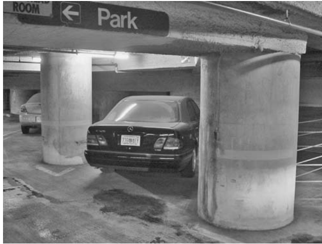
FIGURE 24.22 The huge structural columns of this garage are troubling for security concerns because they are difficult to negotiate with a car, can hide people, and make lighting difficult to accomplish.
