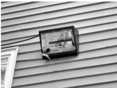
FIGURE 23.1 Broken security light.
