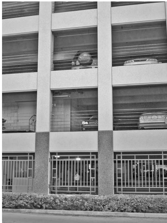
FIGURE 24.7 The ground floor screening was intended to provide security but merely provides a ladder to the second floor. The landscaping and plantings are maintained at a good height for visibility.
