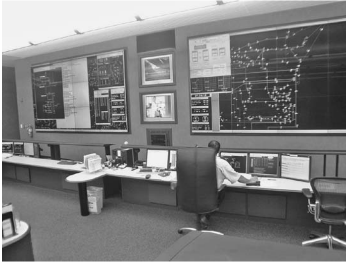
FIGURE 10.9 Control room for power distribution and transmission lines. The lines have to be secure, but so does the control room.
