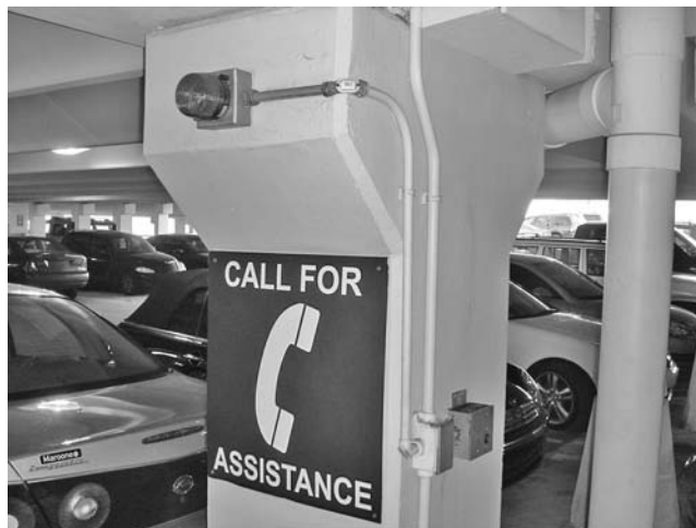
FIGURE 24.14 A personal alarm system should be obvious visually and responded to quickly. This requires preplanning and conduit.
