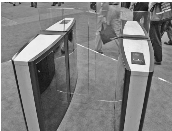
FIGURE 5.10 This hands-free access control has clear panels that prevent persons from piggybacking behind an employee.
