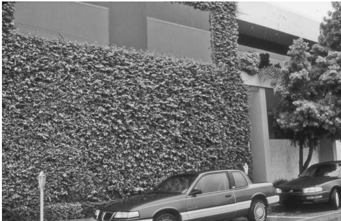
FIGURE 18.32 Living wall removes painting surface.
