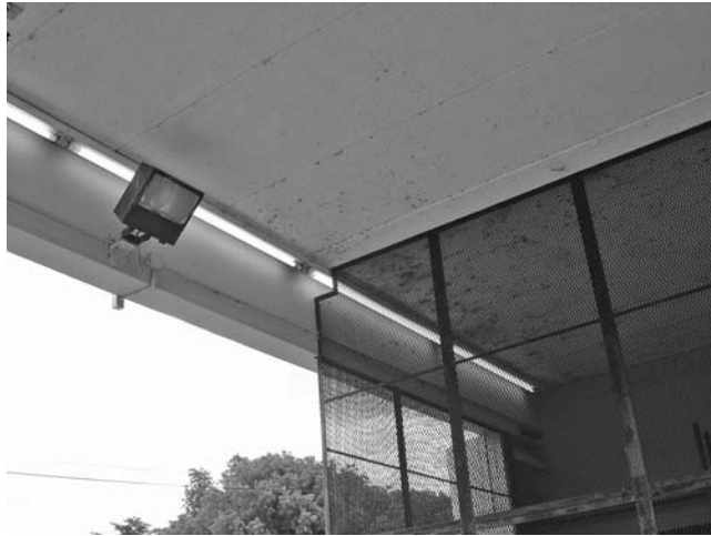
FIGURE 22.12 Exterior fluorescent lights can be used effectively when they are not accessible to vandals and the temperature remains moderate.
