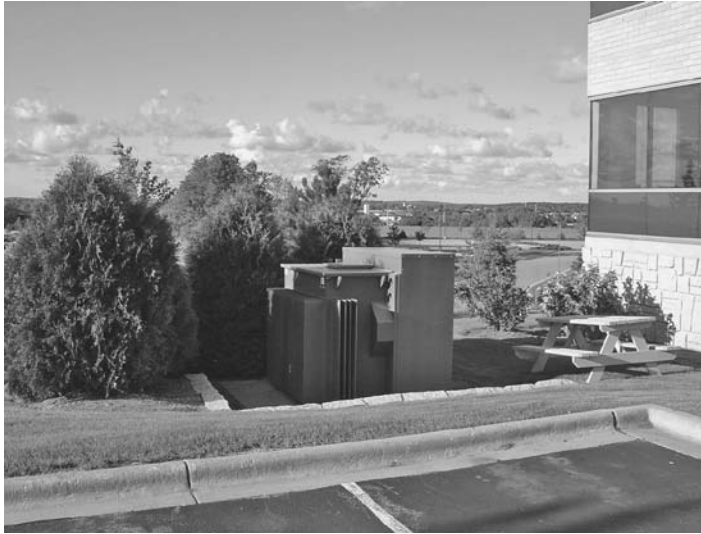
FIGURE 10.11 Transformer adjacent to building façade provides good surveillance but can also act as a hiding place and used as improvised explosive device (IED).
