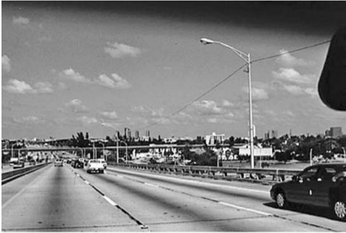
FIGURE 23.3 Street lights along Interstate 95 in South Florida were vandalized by street criminals stealing the copper wiring and rendered unusable. The lights had to be wired on top like a Christmas tree because the wiring was not secured in the bases.
