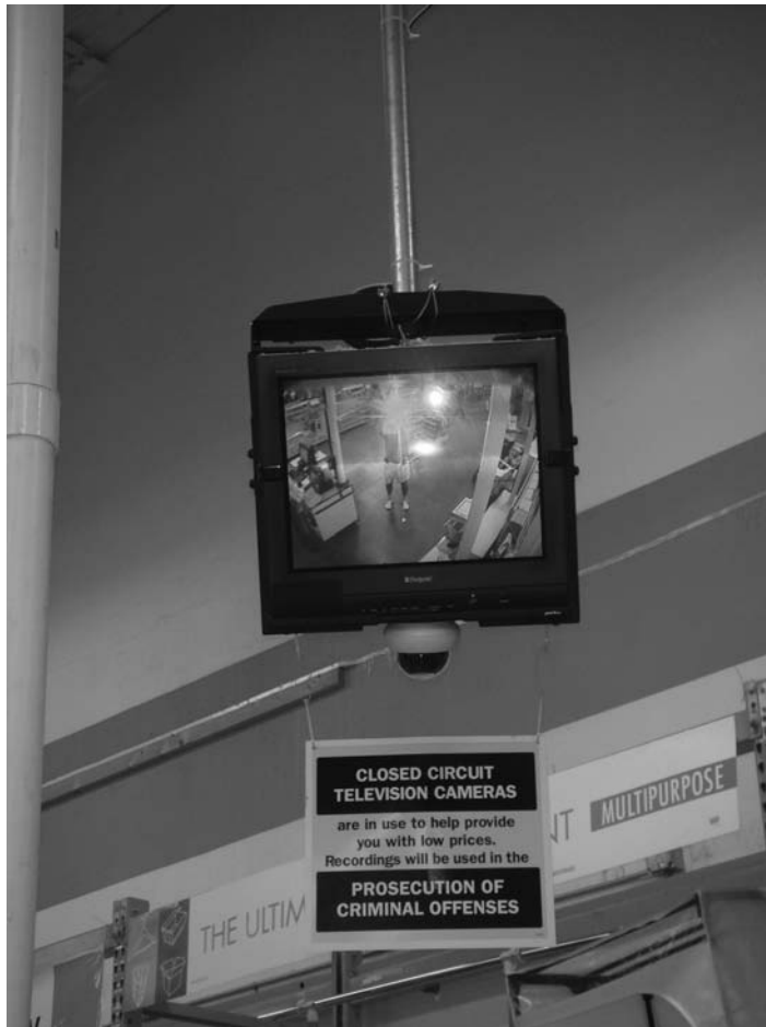
FIGURE 27.7 Cameras and monitors greeting you in an entrance lets the employees and visitors know you are being watched to prevent pilferage and theft.
