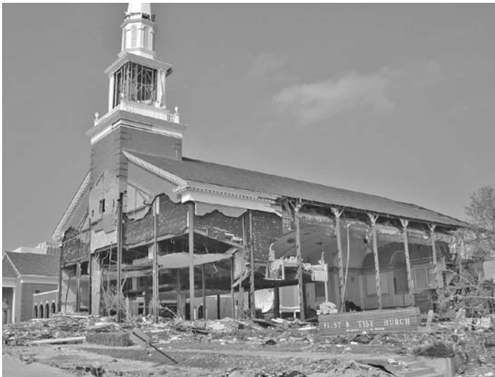
FIGURE 10.20 Gulfport, Mississippi, church damaged by Hurricane Katrina.
