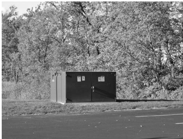
FIGURE 10.10 Transformer sited remotely on grounds. The transformer should be locked and checked for tampering.
