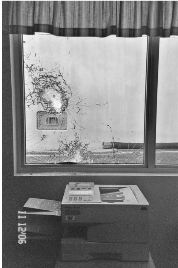
FIGURE 6.5 Hurricane-rated laminated glass provides a security barrier to burglary attempts as well, as this example of an attempted break-in at a county office building demonstrates. The exterior layer of glass broke from the attack, but the interlayer held the glass laminates together and deterred repeated attacks. The glass is intended to stop a 2 × 4 piece of wood from penetrating at 110 mph.
