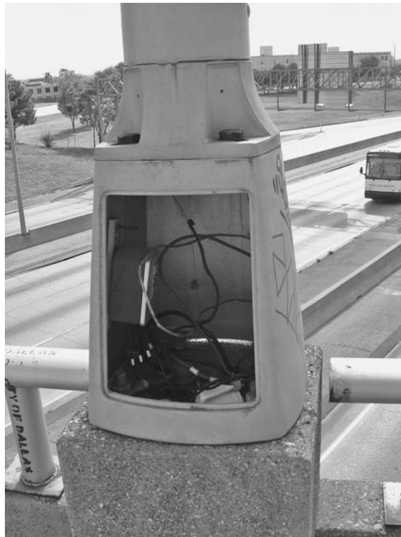
FIGURE 23.4 Open base of light poles vandalized for the copper and aluminum recycling. The lack of security screws on the face plate allowed access to the wiring.
