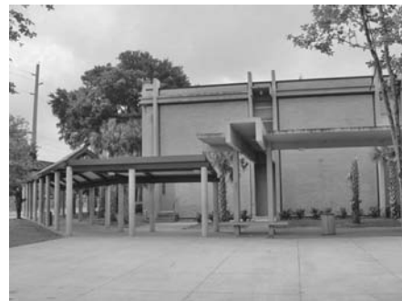
FIGURE 18.7 Catwalks provide an illegal secondary travel path around many schools by encouraging or allowing students to be able to climb on top and gain access to second story windows and roofs.
