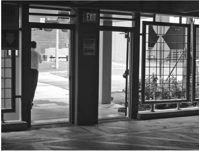
FIGURE 24.4 Ground-level screening of a garage showing defined pedestrian paths. Doors can be locked at night or after hours if needed.
