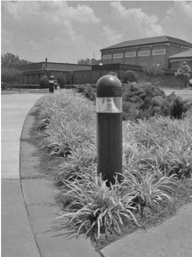
FIGURE 23.19 Pedestrian lighting. Good for preventing trip and falls but ineffective for facial recognition of persons walking toward you.
