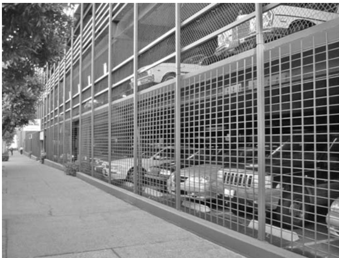
FIGURE 24.5 Ground-level screening and railings have large openings, which create a ladder for someone to climb to the third floor.
