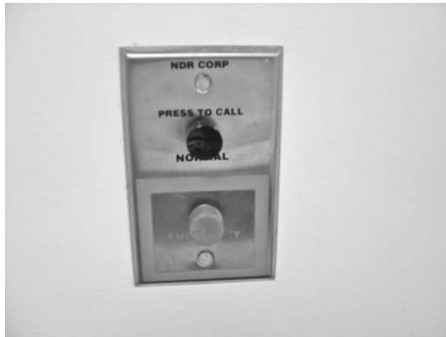
FIGURE 18.44 Duress and panic alarms.
