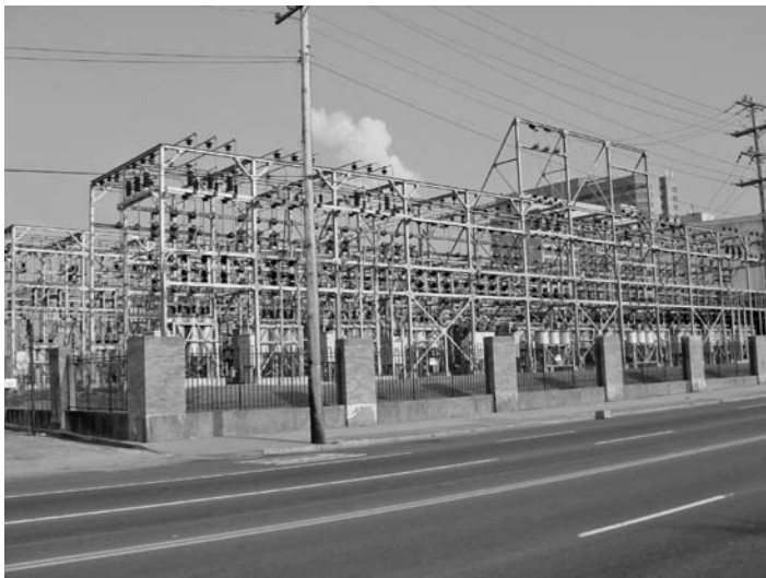
FIGURE 10.12 Electrical substations must be secured from trespassing and tampering.
