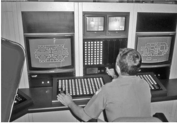
FIGURE 5.4 This control panel is well planned and has favorable human factor operational considerations.
