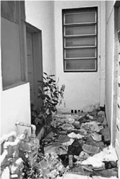
FIGURE 9.15 Trash in a building alcove attracts more garbage and rats.
