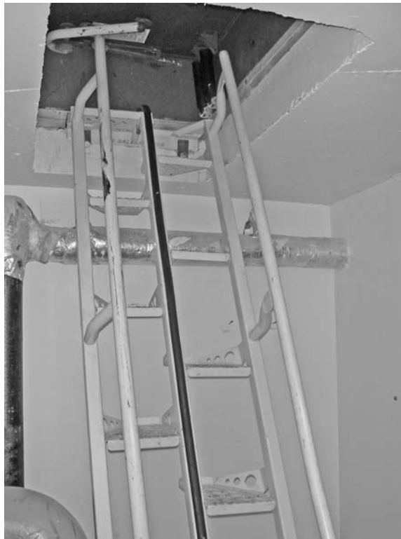
FIGURE 18.40 Secured roof access requires a special stairway and access control.
