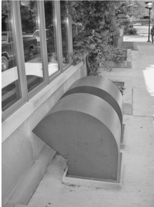
FIGURE 10.16 Air intake vents on the street level are exposed to sabotage.
