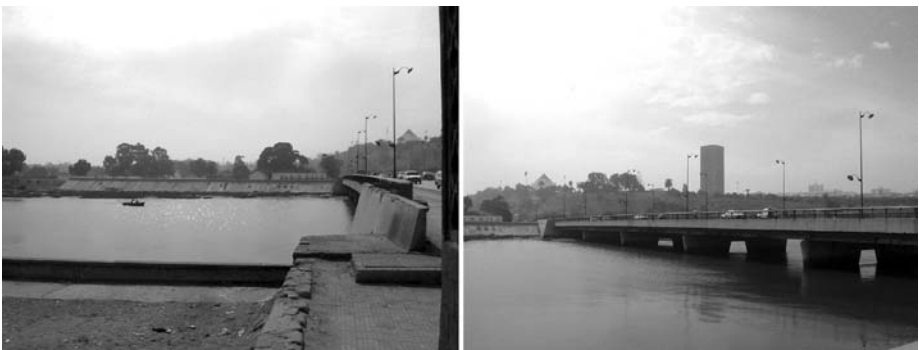
Figure 5.1. Different perspectives of Moulay Hassan Bridge connecting Rabat and Salé over the River Bouregreg. This is a construction dating back to the French colonial period and until the late 1970s was the only road connection between the rival sisters.
