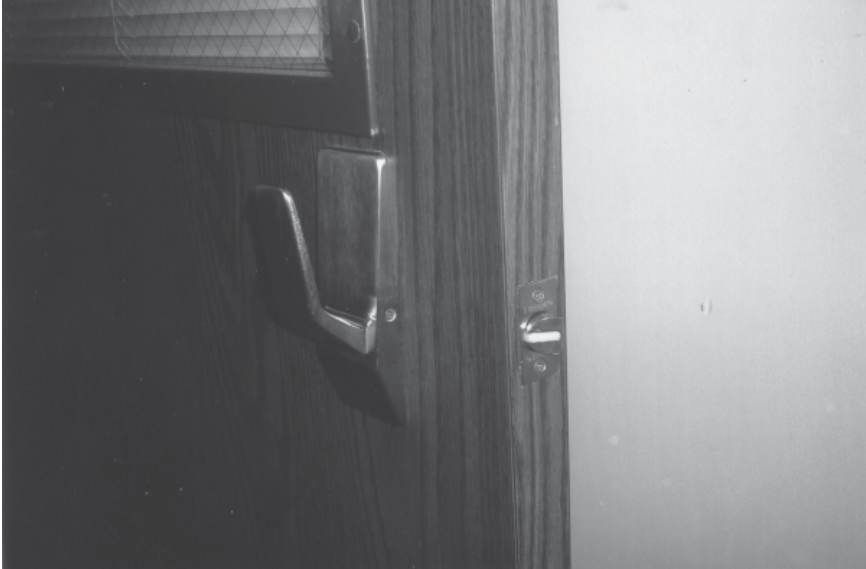
Figure 6-5. Lever Latch. The lever latch works similar to a door knob but the lever has advantages because persons with limited ability to grip a doorknob or operate at thumb latch. This photo shows a door to a patient room in a hospital. (Photo by Robert Reid, 2004)
