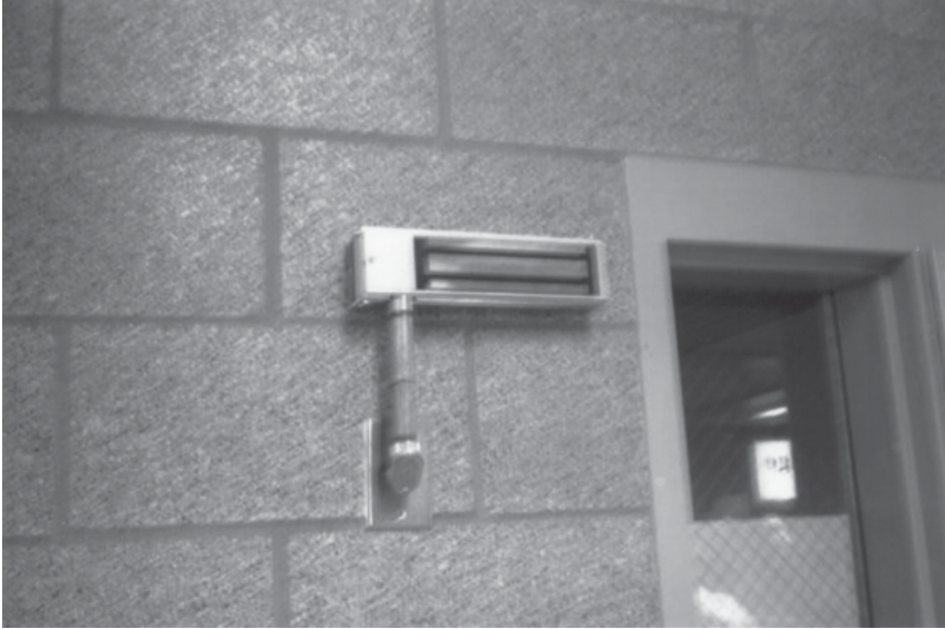
Figure 7-1. Electromagnetic Lock. This electromagnetic lock is being used in a school to hold doors open. The device can also be mounted to hold the door closed. (Photo by Robert Reid, 2004)
