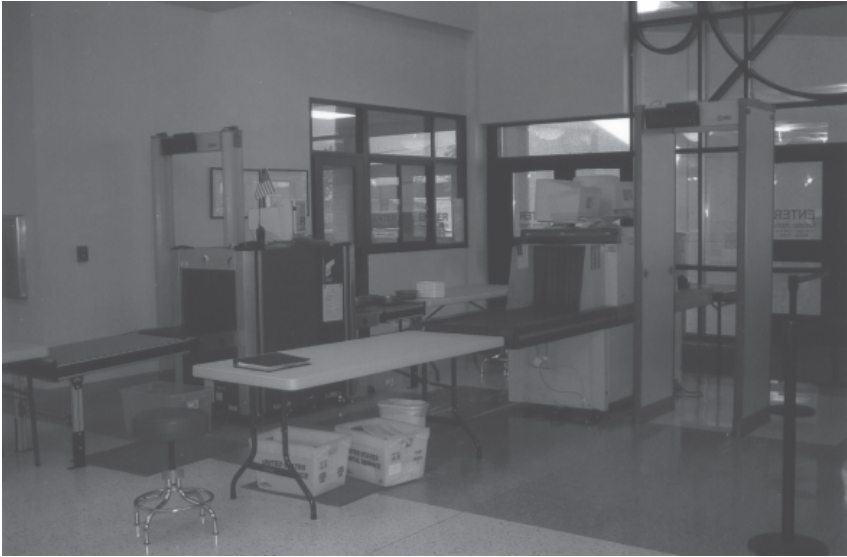
Figure 8-6. Metal detector station. (Photo by Robert Reid, 2004)
