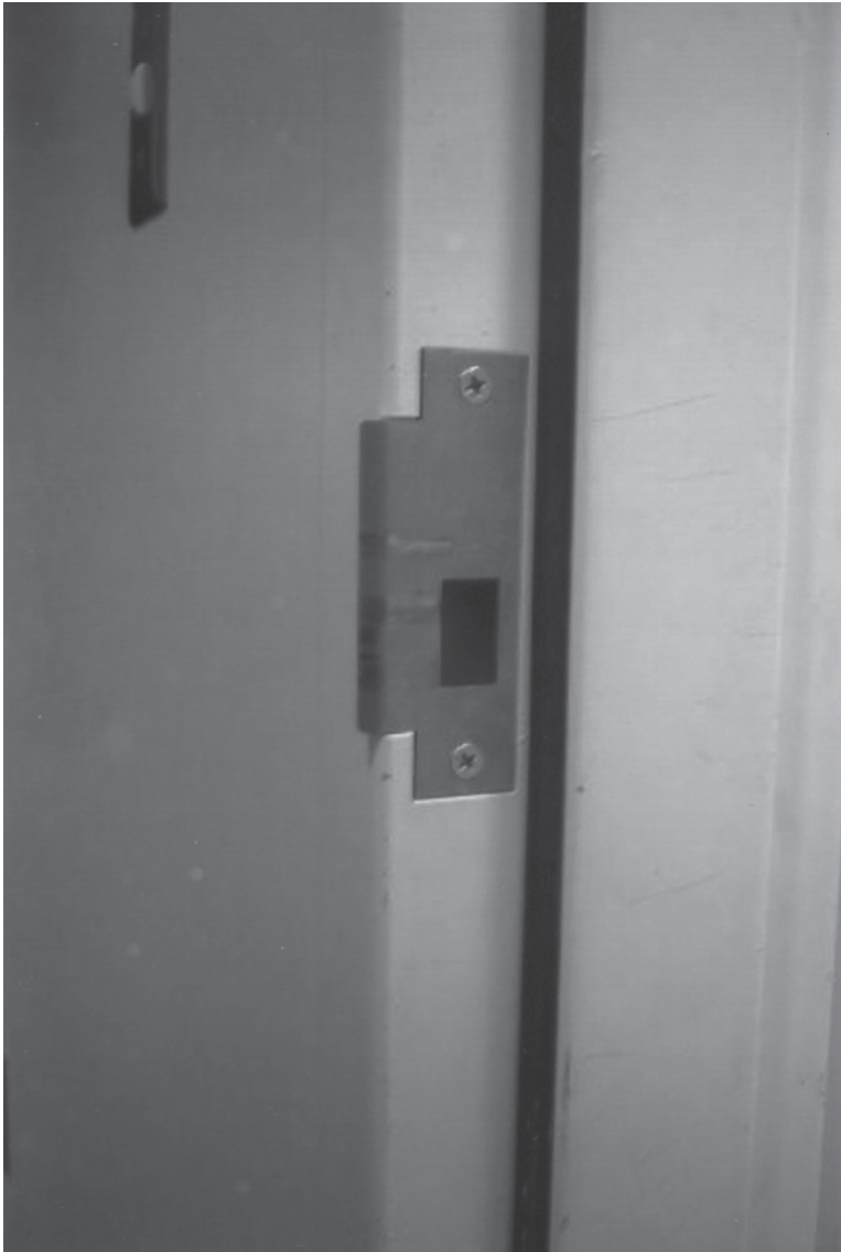
Figure 6-1. Strike and Strike Pocket. The edge of the jamb where the door closes is called the “strike.” The metal hole in the door that catches the latch is called the “strike pocket.” (Photo by Robert Reid, 2004)
