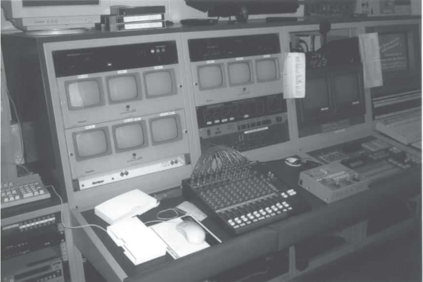
Figure 11-5. CCTV camera monitoring station. (Photo by Robert Reid, 2004).
