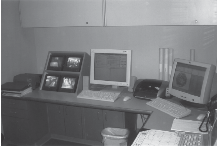
Figure 9-3. Control room station. (Photo by Robert Reid, 2004)
