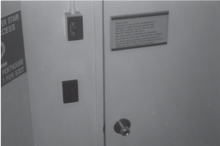
Figure 8-3. Proximity Reader. This photo shows a typical proximity reader installed in a stairwell of a hospital. The secured area is the maternity ward. (Photo by Robert Reid, 2004)
