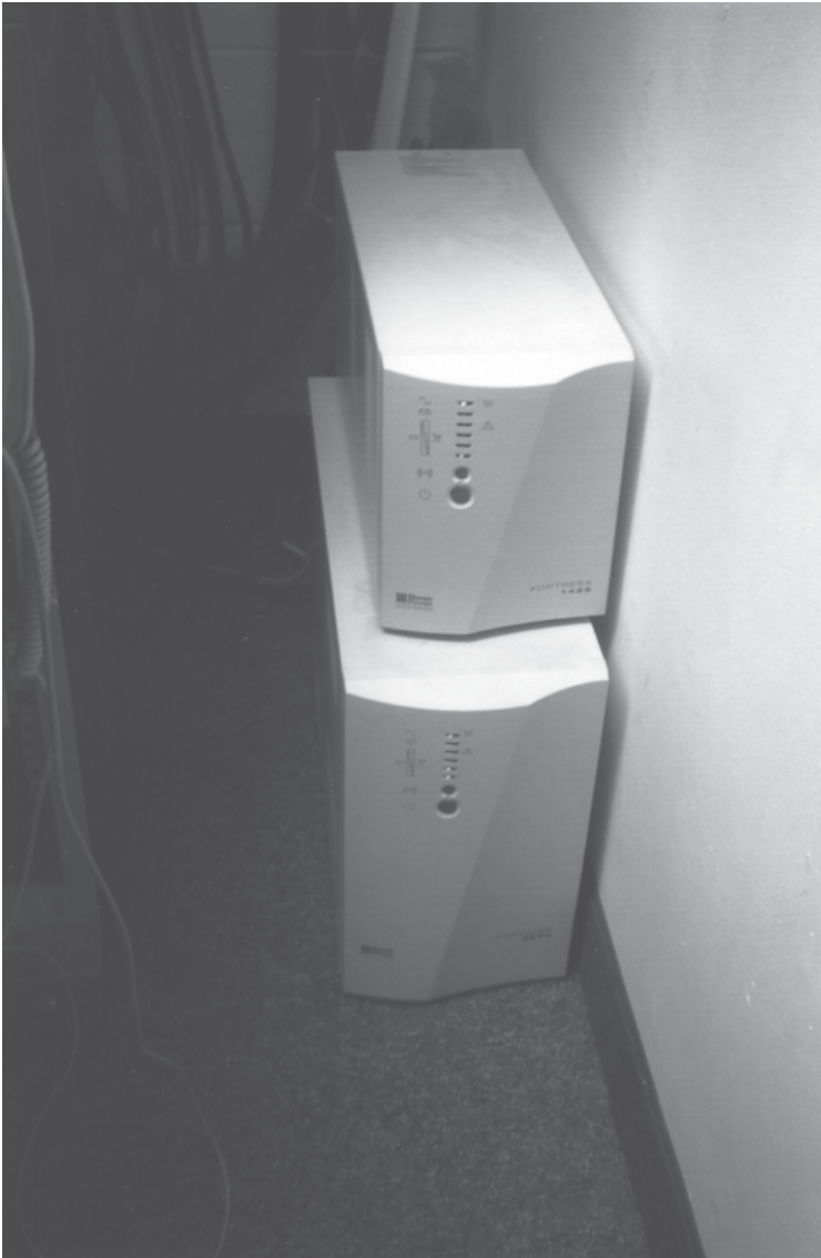
Figure 13-3. UPS system. (Photo by Robert Reid, 2004).
