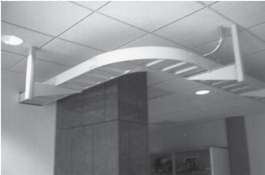
Figure 13-1. Cable tray. ( Photo by Robert Reid, 2004. )
