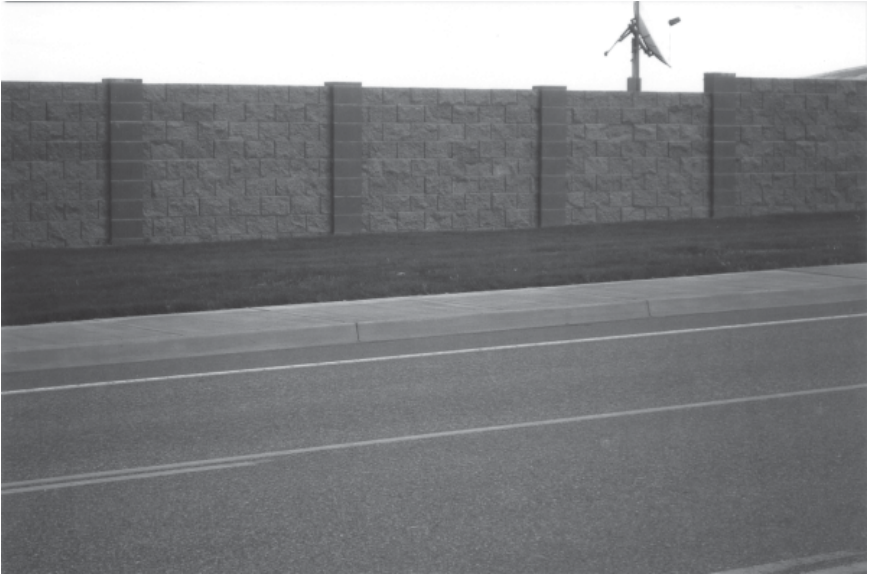
Figure 3-9. Block walls provide good perimeter security, but they are expensive. (Photo by Robert Reid, 2004)
