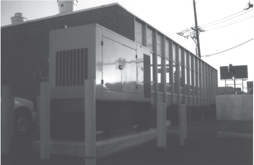
Figure 13-2. Emergency generator. (Photo by Robert Reid, 2004).
