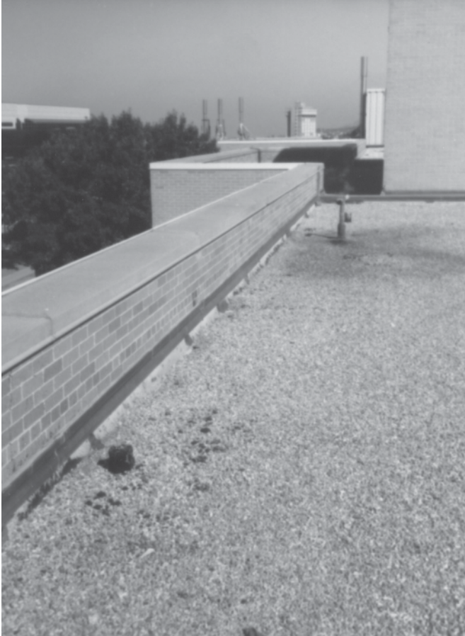
Figure 4-1. Parapet wall. The problem with this type of wall is that the wall can catch explosive devices that will fall off of a sloped roof. (Photo by Robert Reid, 2004)
