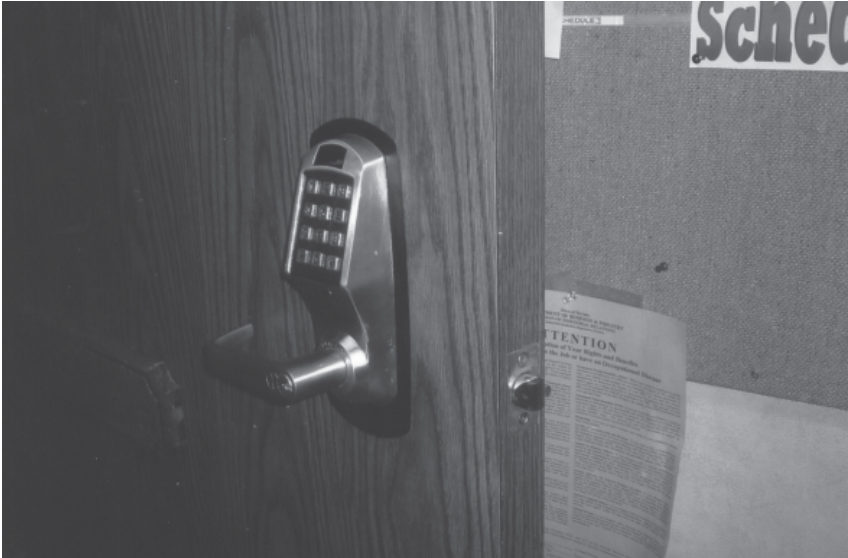
Figure 7-4. Battery powered combination door lock. (Photo by Robert Reid, 2004)
