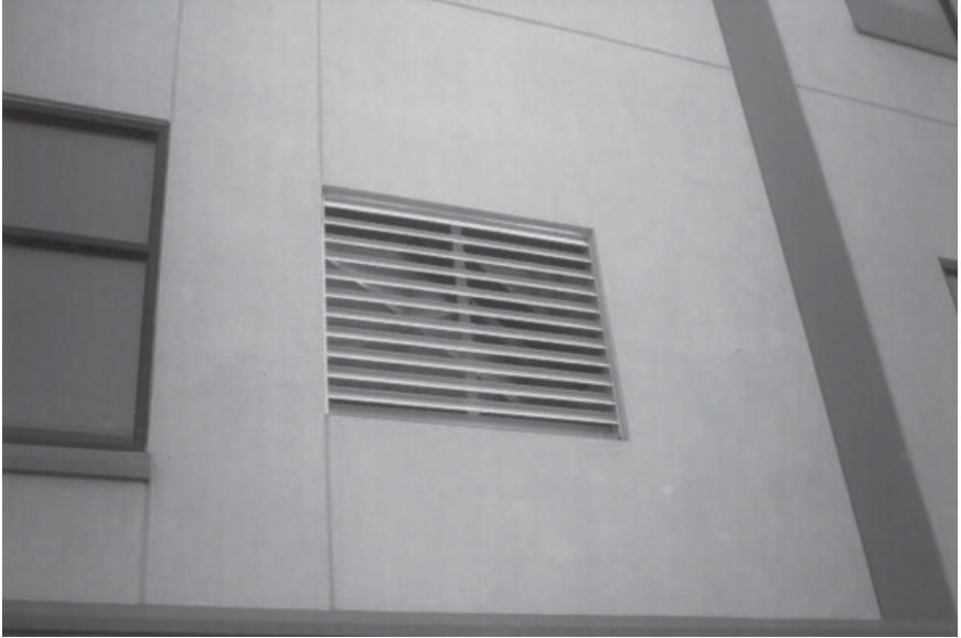
Figure 5-9. Ventilation opening for an office building. While many building ventilation openings are for the roof, or below ground with a grille, some facilities continue to have ventilation openings on the side of the building. (Photo by Robert Reid, 204)
