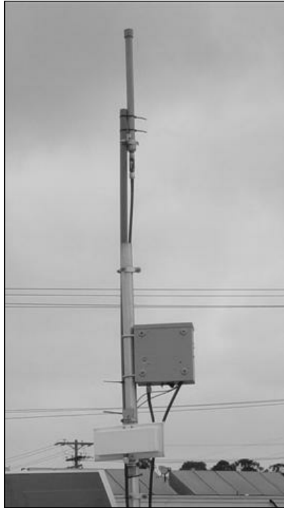
Figure 12.17 2.4-GHz and 5.8-GHz Antennas Mounted to a Structure
