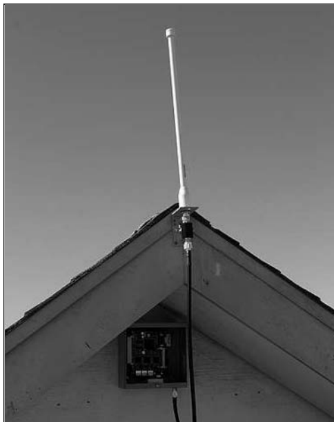
Figure 11.16 L-shaped Bracket-mounted Antenna with an Eave-protected Enclosure
