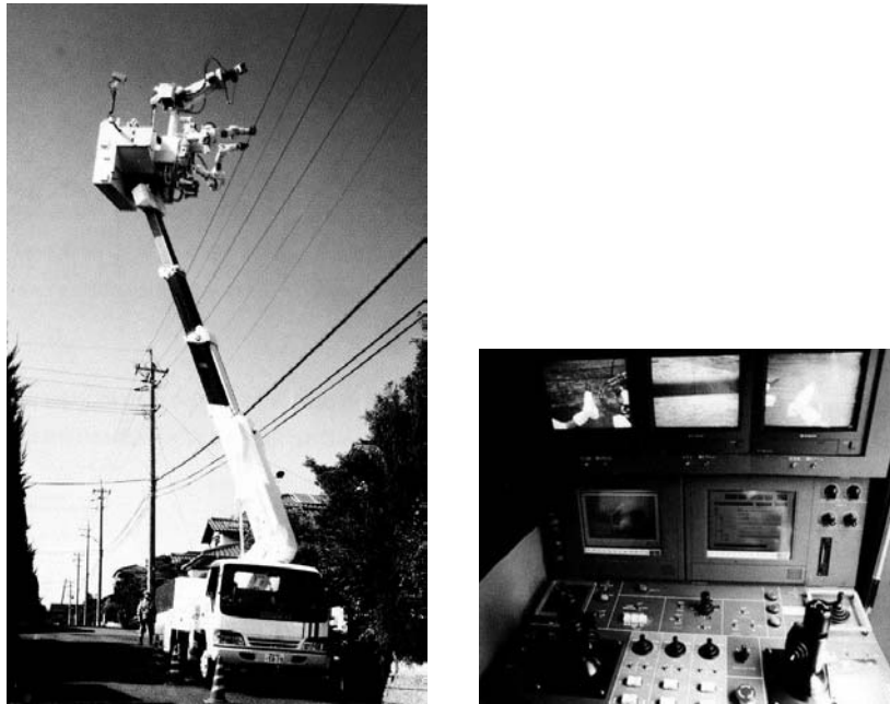
Figure 15.9: The “Hot-Line Telerobot System” from Kyushu ELeetric Power Co. A teleoperated robot repairs a high-voltage power line (left). The operator’s interface to the system (right). (Courtesy of Blake Hannaford with permission of MIT Press. Reprinted from K. Goldberg, The Robot in the Garden , Cambridge, MA: The MIT Press, 2000.)
