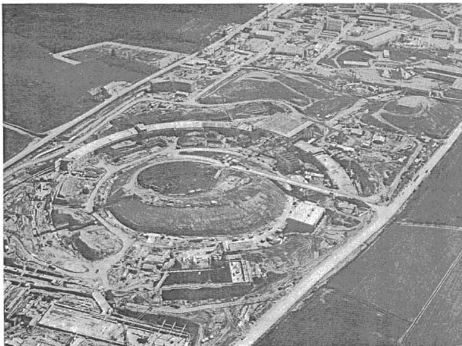
Fig. 7.25 State of construction in April 1969. In the foreground, work has started on the building housing the control room, and also on the Experimental Hall 14 . To the right, Octant 3 is already being covered and the tunnel is complete as far as Octant 7 . On the far side, the steel work for Hall 11 is in position and in the background the tunnel of the booster is about half complete. Top right is the PS itself. (Courtesy of CERN).
