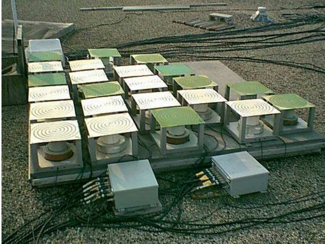
Fig. 1. The antenna array. Elements rest on a platform covered in fine wire mesh which serves as a larger ground screen. Each of the two gray boxes in the foreground contain line amps for 8 antennas (a third box is located on the far side of the array). The base of the calibration source mast is visible in the upper left. One of the 23 elements shown is currently not working.
