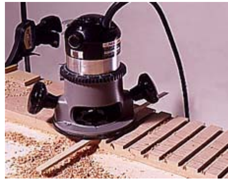
7--The dentil molding is cut using a router with a guide strip screwed to its base. The strip rides in the previously cut dado.
