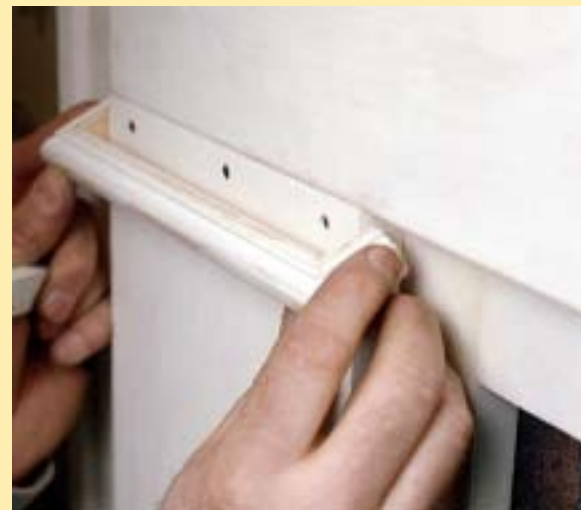
A preassembled band of molding can be gently coaxed into place—while the miter remains tight.
