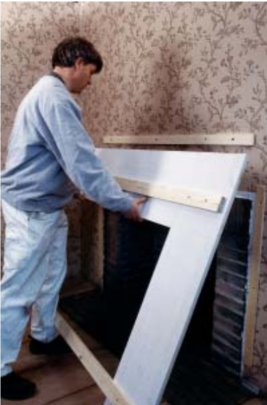
Position the braced foundation against the furring strips. Make sure it's plumb and leveled, then screw it to the strips with #8 by 1½-in. wood screws.
