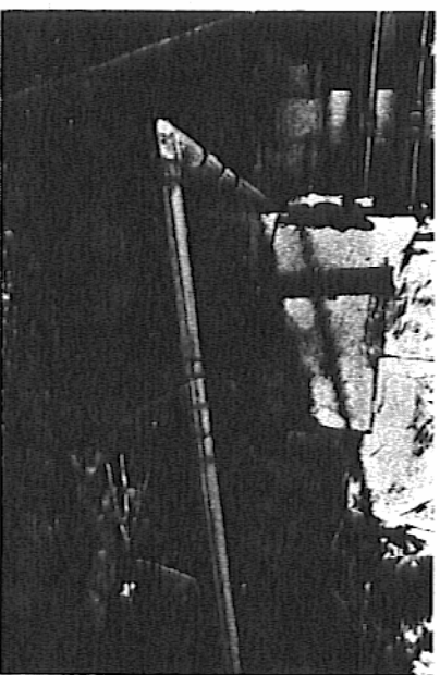
At the bridge support, the cable comes out of the ground, crosses over the water along the bridge and then reenters the ground on the opposite bank.
