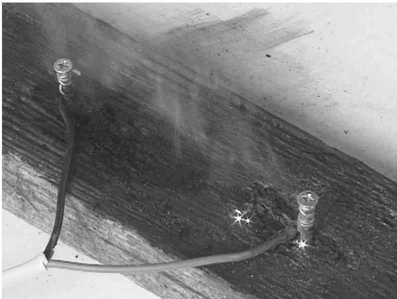
Figure 3.15 Tracking through wet wood at 230 V AC. Mini arcs can be seen within the wet wood. Dark areas show where carbonisation of the wood has already occurred (Photo: APU/LFB)
