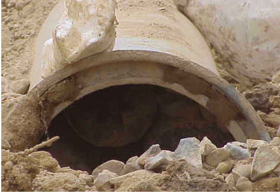
Projectiles inside of a roadside culvert pipe
