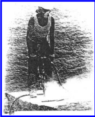
(a) Drilling using hand held Rock drill. It is slow, tedious, noisy and not very productive.
