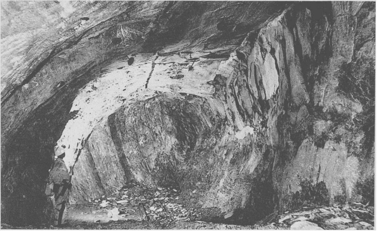
Figure 10.14: Spalling around a tunnel in massive quartzite at a depth of 2,700 m below surface in a South African gold mine. Photograph provided by Mr David Ortlepp.
