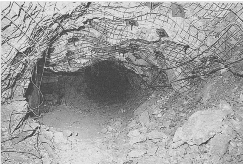
Figure 11.12: Roof deformation and sidewall failure in a drive in the 500 copper orebody in the Mount Isa mine in Australia. Closure between the roof and floor is more than 2 m but the rockbolts and weldmesh have prevented total collapse. After Mathews and Edwards (1969). Mount Isa Mines photograph.
