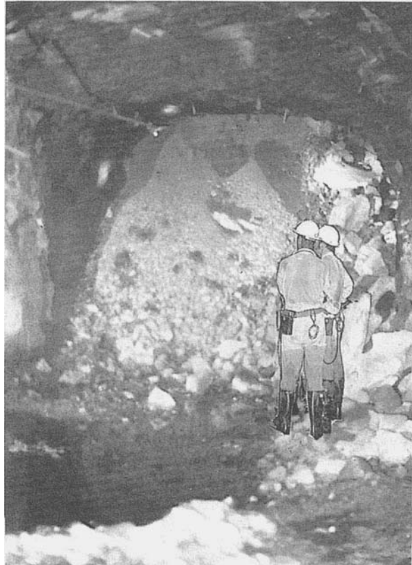
Figure 11.7: Drawpoint reinforced with cement grouted untensioned rebar, installed during development of the drawpoint.
