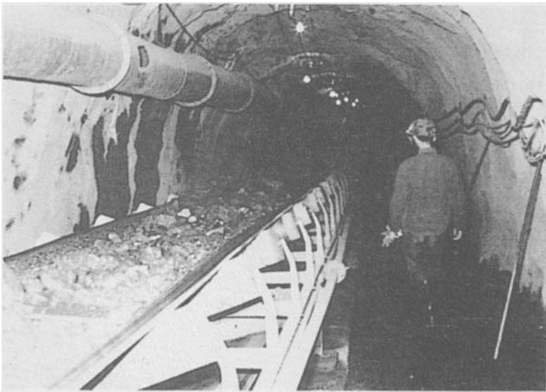
Figure 11.2: A conveyor tunnel with grouted rockbolts and shotcrete support. Here the tunnel has been designed for a life of about ten years and possible corrosion of the support system was a major factor in the choice of the support.
