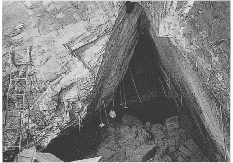
Figure 6.3: Failure of a wedge where the rockbolt support was inadequate.
