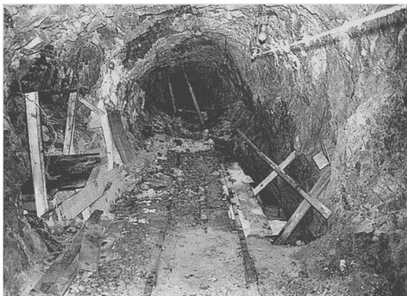
Figure 11.3: An accumulation of small blocks and wedges which have fallen from the roof and walls of an unsupported tunnel in a closely jointed rock mass. These small failures, induced by mining activities in adjacent stopes, could be controlled by the installation of light support systems such as those illustrated in Figures 11.1 and 11.2. A layer of shotcrete can provide very effective support for this type of rock mass.
