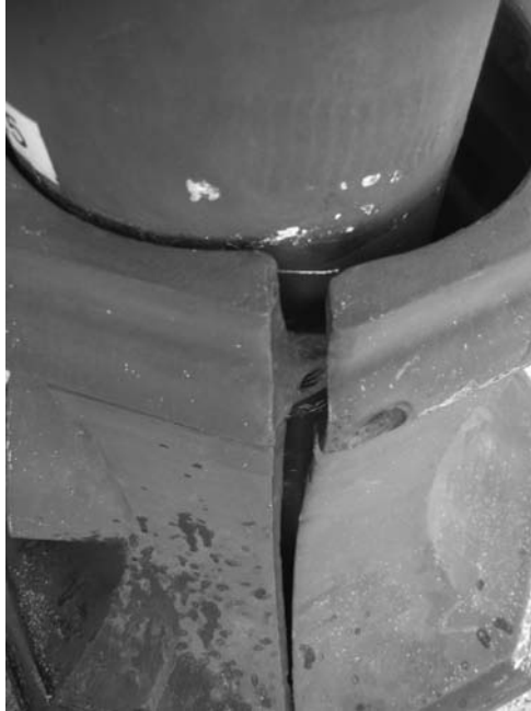
FIGURE 7.5 (See color insert following p. 142.) Corrosion observed around a bolt joint.
