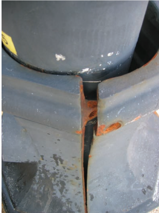
FIGURE 7.5 Corrosion observed around a bolt joint.
