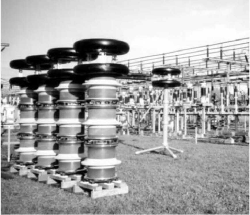
Figure 2.22 Modular reactors of a series resonant circuit with variable frequency during an on-site test of very long polymeric cables (courtesy FKH, Zurich, Switzerland)
