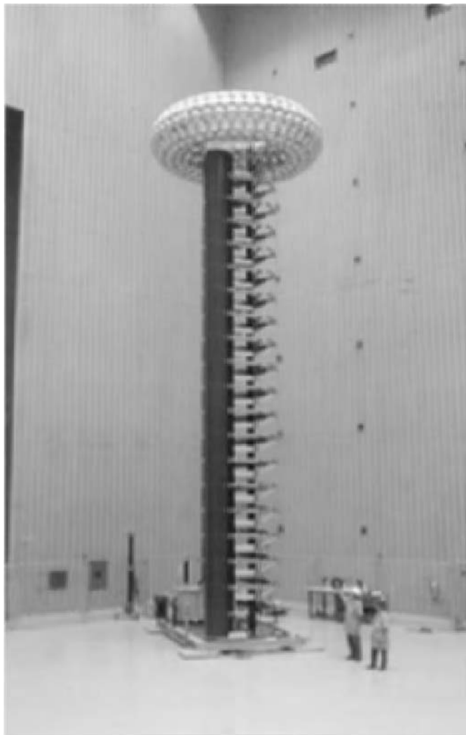
Figure 2.34 Indoor impulse generator, 20-stage, 4-MV, 200-kJ, with encapsulated sphere gaps (courtesy of CEPTEL, Rio de Janeiro, manufactured by Haefely)
