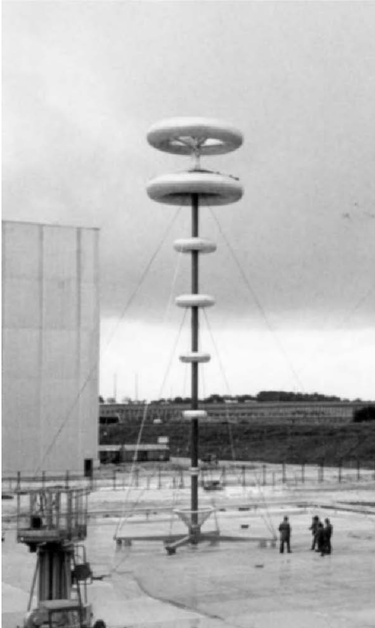
Figure 3.41 Series-damped capacitor voltage divider for 6-MV impulse voltage (courtesy EdF, Les Renardieres, France)
