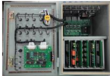
Fig. 6. Interior configuration of monitoring device
