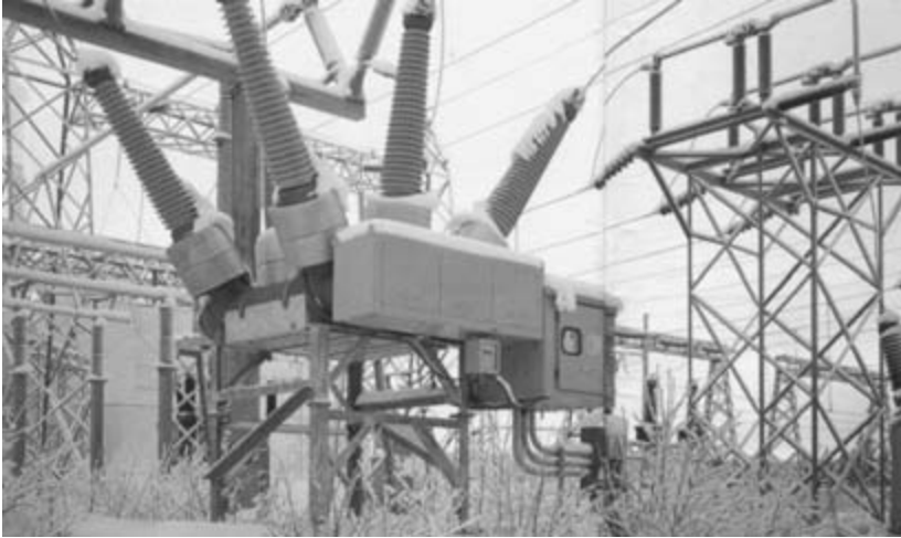
Figure 9.17 Outdoor installation of 145 kV dead tank switchgear in the USA (courtesy ALSTOM T&D Ltd)
