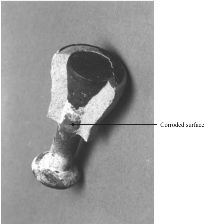
Figure 6.4 Corroded pin (with some mortar removed)
