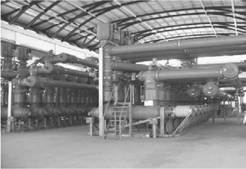
Figure 2.7 A modern 400 kV GIS
