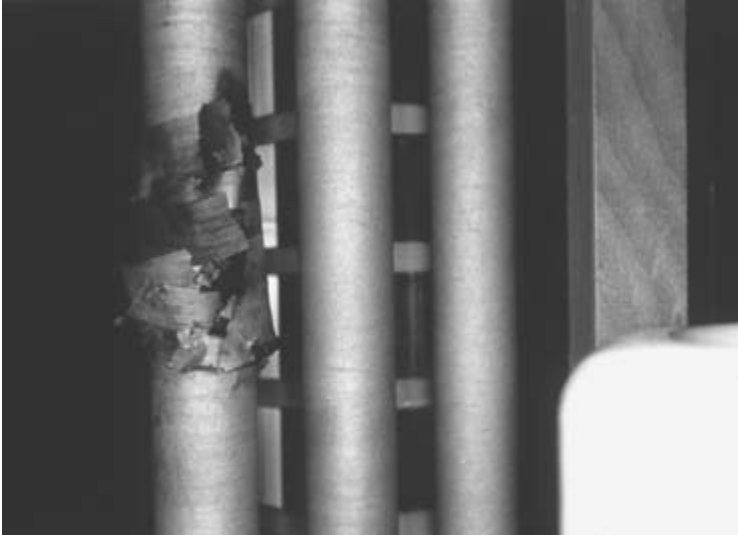
Figure 11.1 Insulation rupture of the neutral lead (courtesy of ALSTOM T&D – Transformers, Stafford (TST))
