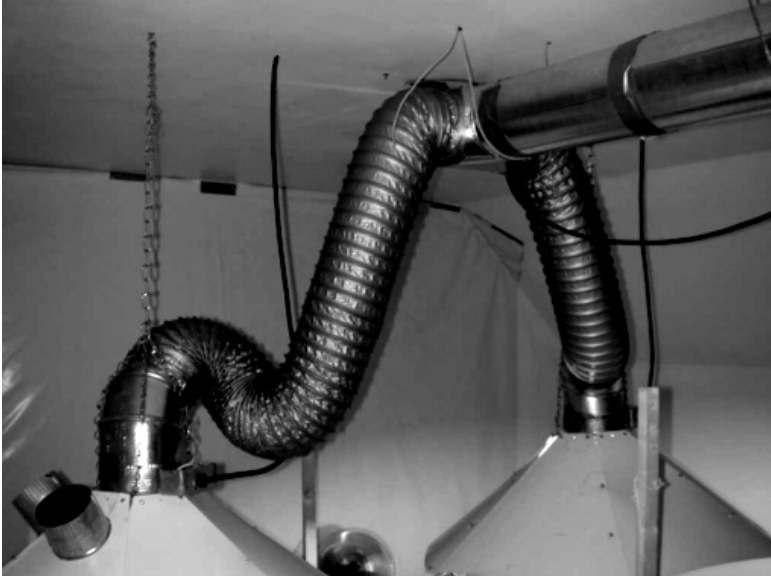
Figure 5.12 - This picture shows two air-cooled hoods attached to their respective air ducts. This photograph is by Chimera.
