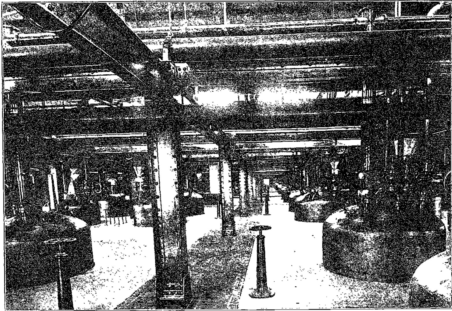
AUTOCLAVES IN WHICH AMMONIA GAS IS PRODUCED
